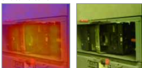
Normal operating temperature on mission critical breaker
